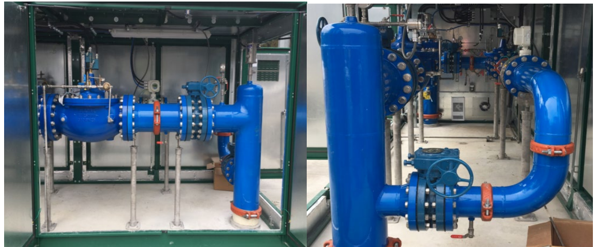
Figure 12: Norum Road PRV Station
