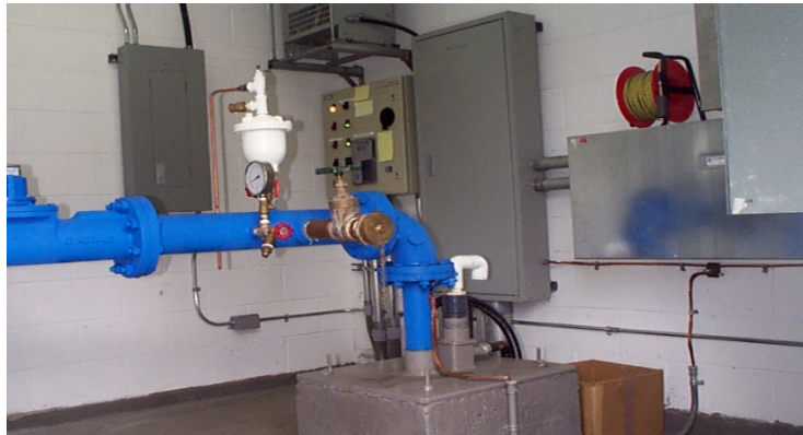
Figure 17: Well #1, Watershed Park Wells
