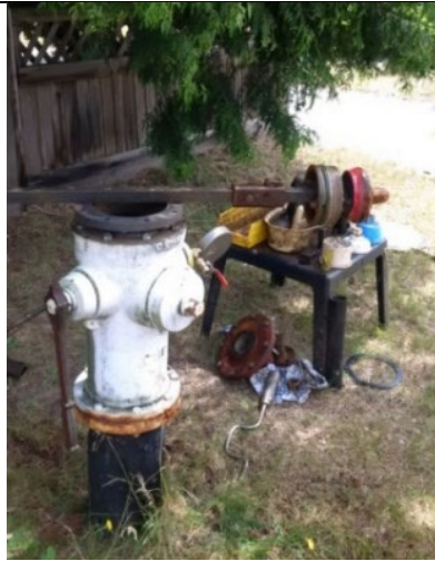
Figure 15: Fire Hydrant Undergoing Regular Annual Maintenance
