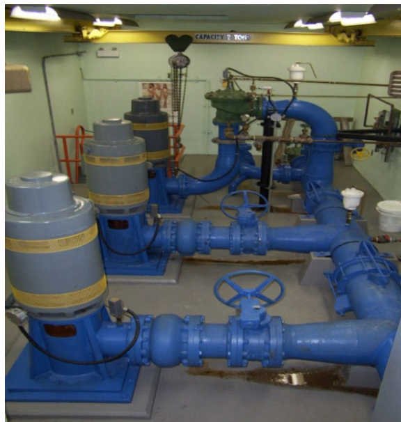
Figure 10: Pump Station on 4 Avenue at Pebble Hill Reservoir
